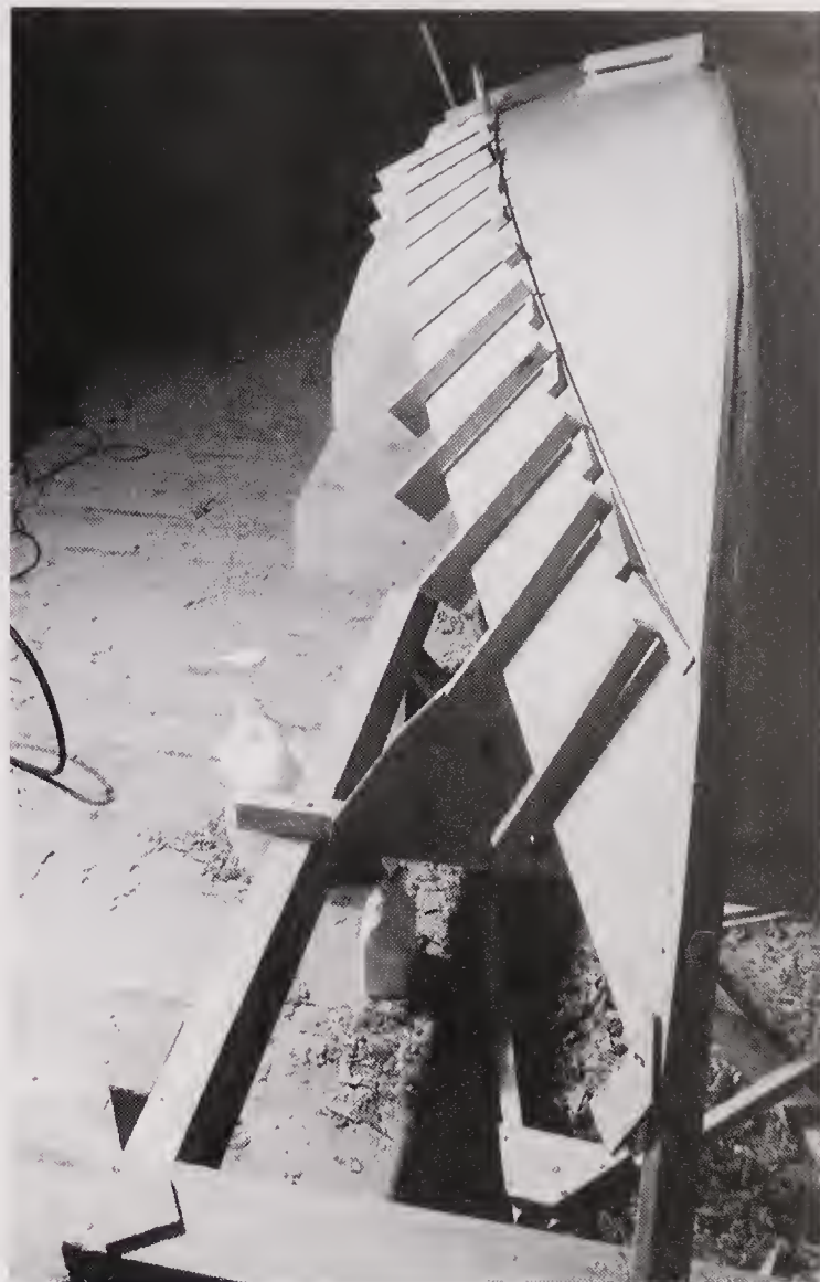
Planks are glued in place. 3 or 4 clamps are loosely positioned; the wedges just tight enough to keep the clamps in place. Check all round to make sure the plank is correctly placed. Then fit all the clamps in the same way, then push all the wedges home. Fit the clamps and wedges just clear of the inner edge, so it will be easier to clean up the glue.
