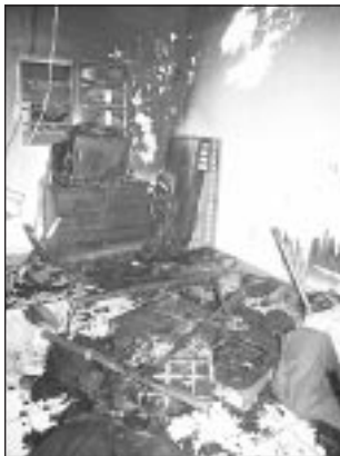
This bedroom was burnt by fire which officials said was caused by a faulty fan.
